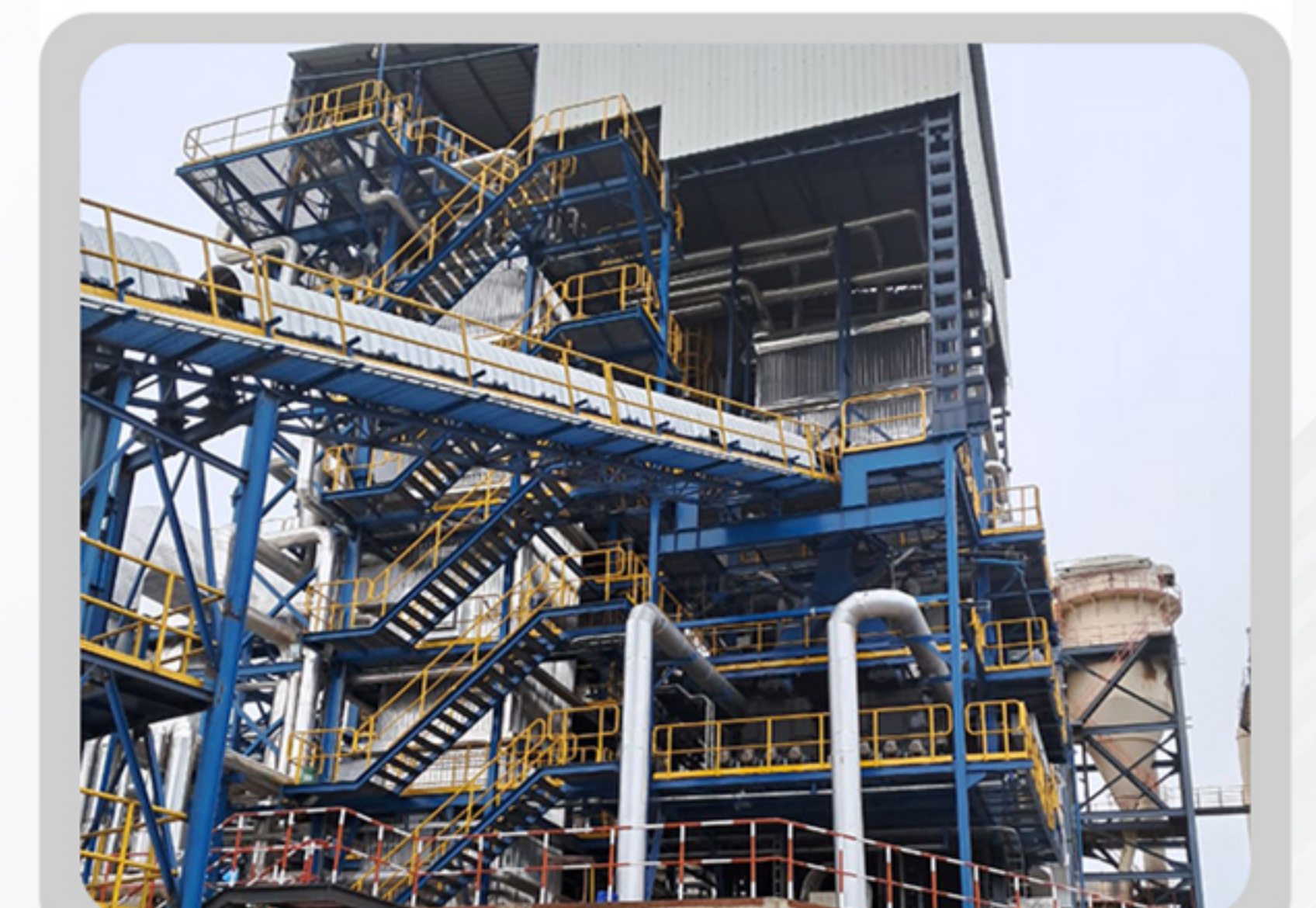
31 MW Energy Plant for an MDF Industry in North India
