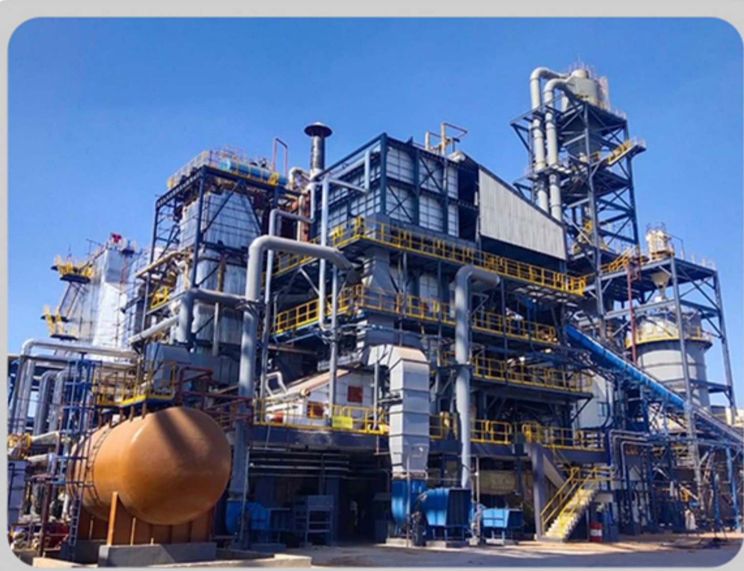
64 MW Energy Plant for an MDF Industry in West India
