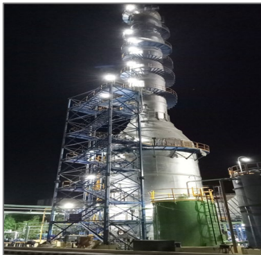
Commissioned a flue gas desulphurisation (FGD) system for a WHRB of a carbon black company in Goa, India
