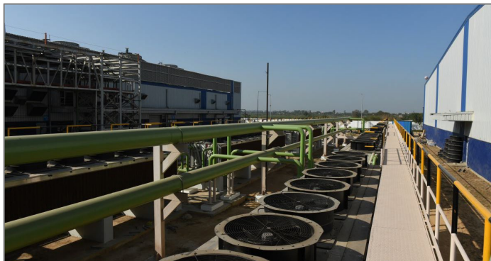
Commissioned an adiabatic dry cooler of 813 kW for a beverages major in Uttar Pradesh, India
