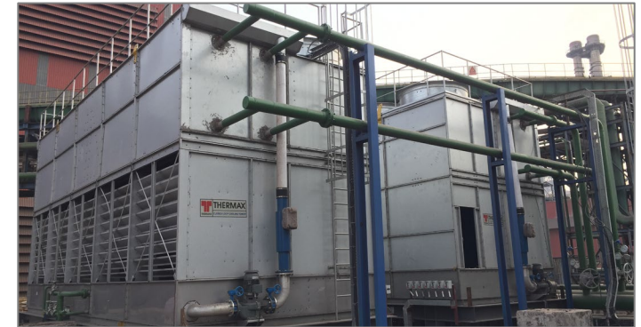
Three units of closed loop cooling towers installed at a steel major at Odisha, India
