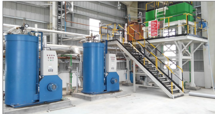
Two units of Revomax deployed at an FMCG major in Assam, India
