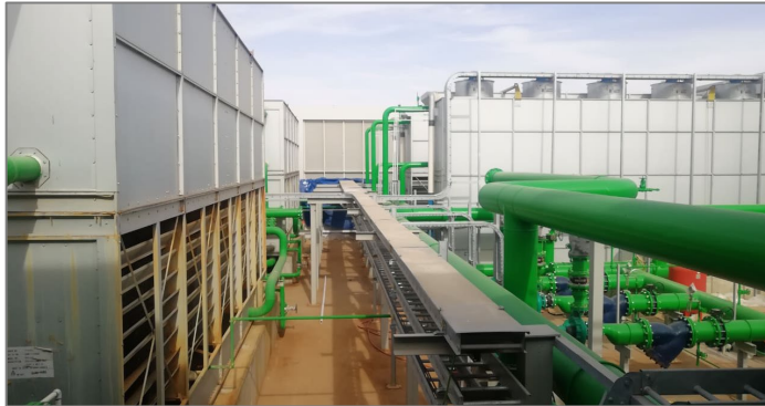
Installed a closed loop cooling tower of capacity 360 CMH at a beverages major in Saudi Arabia
