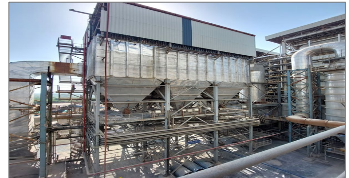
Commissioned a flue gas cleaning system (FGCS) for a municipal solid waste-based waste-to-energy power plant in Delhi, India
