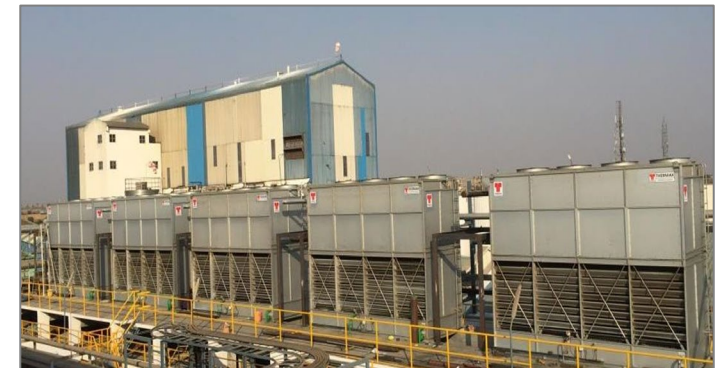
Five evaporative condensers of 550 TR each installed for a dairy major in Maharashtra, India
