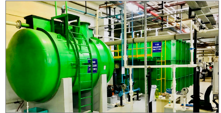
Installed a bioCask based STP for an engineering multinational in Maharashtra, India
