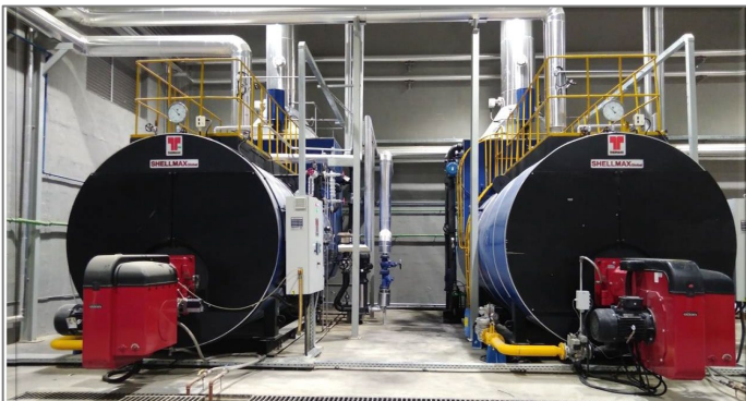
2 X 8 TPH of Shellmax Global boilers deployed at a dairy major in Saudi Arabia
