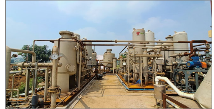
Commissioned a pressure swing adsorption based biogas purification system for a 10 TPD bio-CNG plant in Uttar Pradesh, India
