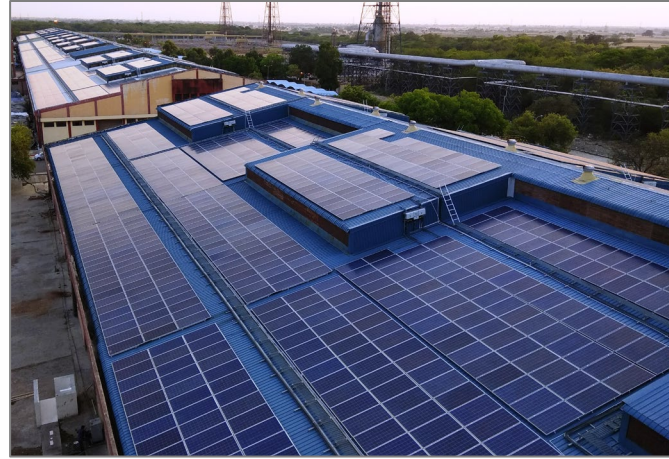
A 5.76 MW, largest single roof solar PV plant installed at one of the largest petrochemical complexes of Government of India's 'Navratna' company
