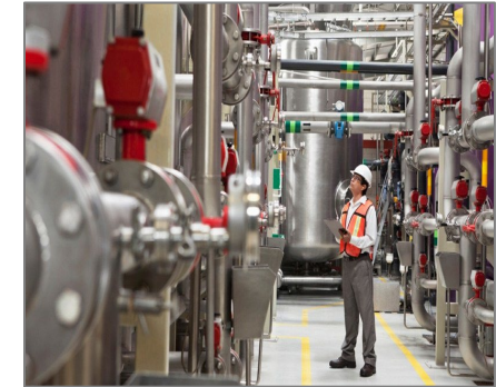
O&M for a 54 MW waste heat recovery power plant for a cement major in Rajasthan, India
