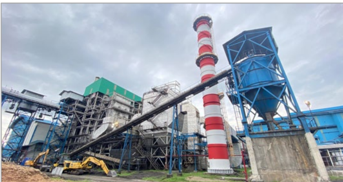
Supplied 2 X 120 TPH biomass boilers for a leading sugar producing company in Indonesia
