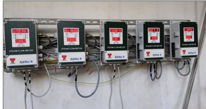
Installed steam flow meters for a dairy major in Tamil Nadu, India
