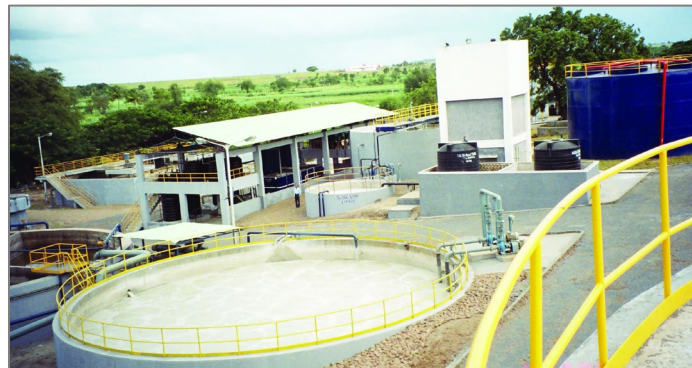
An effluent treatment plant installed for a dairy major in Maharashtra, India
