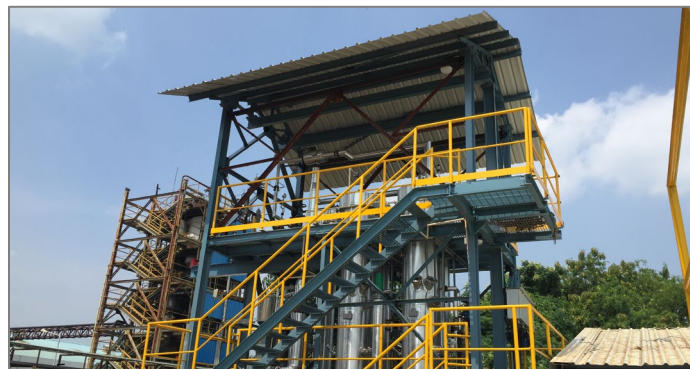
Commissioned a zero liquid discharge (ZLD) plant at a polyester company in Maharashtra, India
