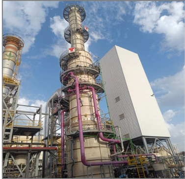
Commissioned a flue gas desulphurisation (FGD) system for a sugar refinery in Saudi Arabia
