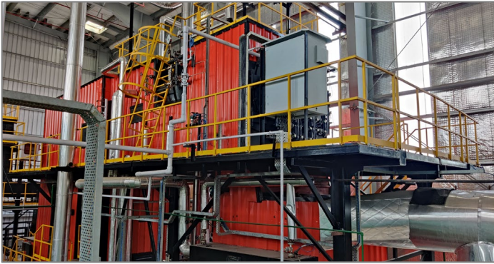
Supplied biomass based steam for a tyre major in Maharashtra, India
