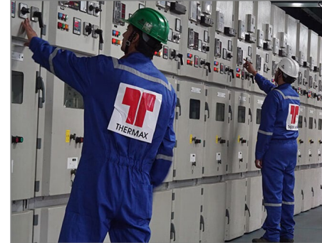
O&M for a 60 MW captive power plant for an oil and gas company in Rajasthan, India
