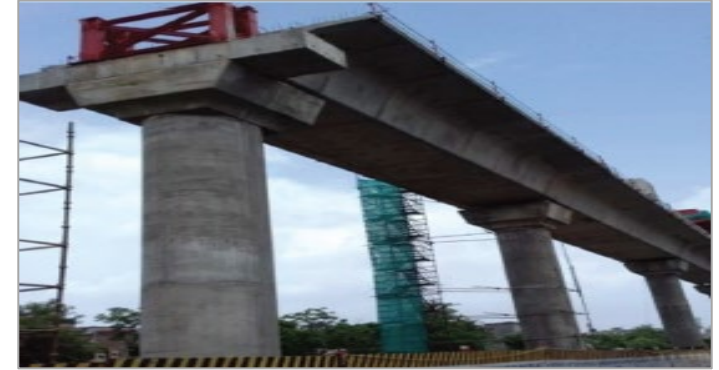
Supplied Neutrol® range of admixtures for an esteemed metro project in India
