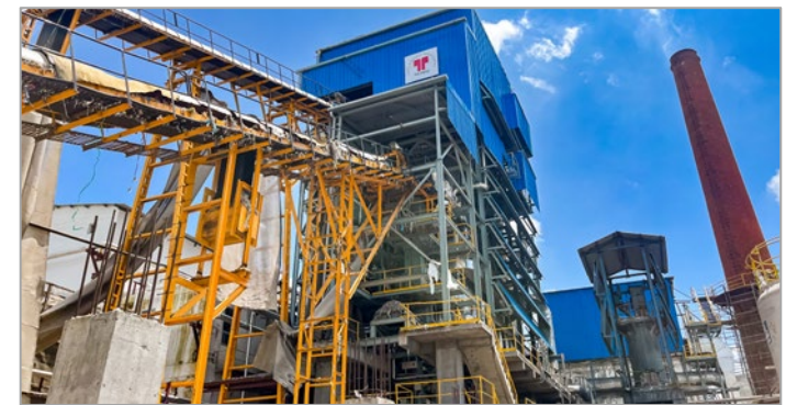
Supplied 40 TPH waste to energy boiler firing non-recyclable solid waste and refuse derived fuel for a leading paper mill in North India
