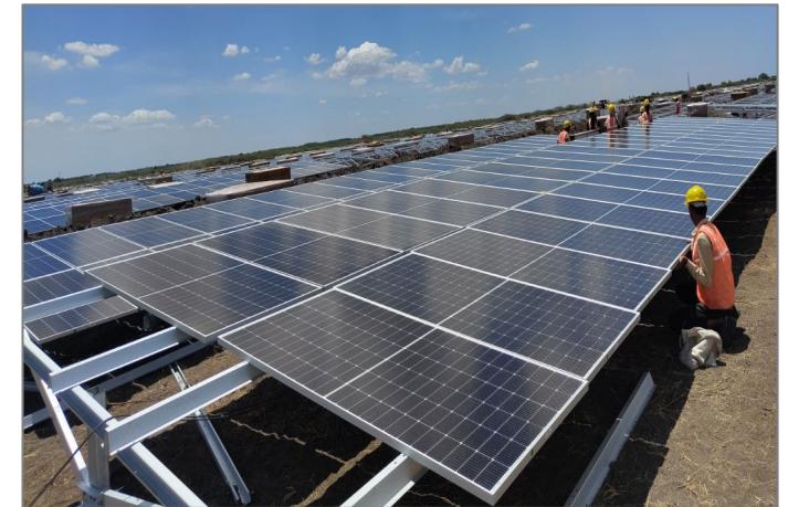
A bundled project of 90 MWp solar and 39 MW wind commissioned in Tamil Nadu, India
