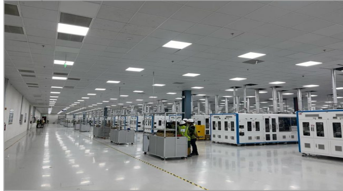
Commissioned a process exhaust system for solar PV cell and modules production lines for a power company in Tamil Nadu, India
